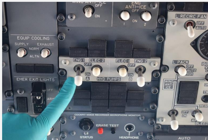
Figure 14: The electrical hydraulic pumps found in the “OFF” position during the field investigation.
