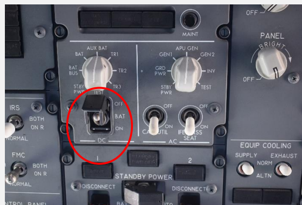
Figure 12: The battery power switch found in the "OFF" position during the field investigation.
