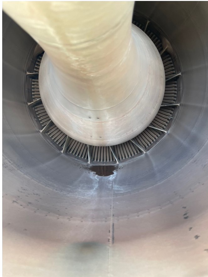
Fig 4: Excess pool of liquid sitting in the bypass duct, as seen from the aft
